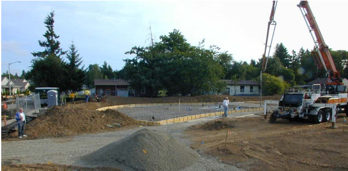
This view of Ball-Michel Park was taken during construction in 2006, looking from near the corner of S.E. 56th and Firwood towards the area to be occupied by the climbing apparatus.
