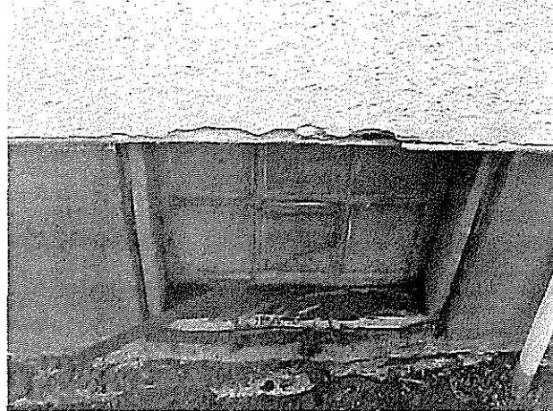
Sample of a deteriorated basement window.
