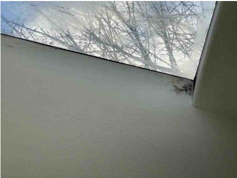
Black Mold Bathroom Skylight
