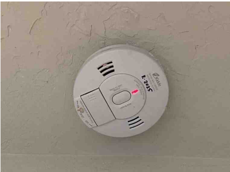
Smoke/Co Det Sample
