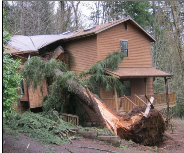
Windstorm damage – March 13, 2011
