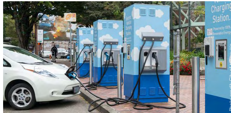
Electric vehicle charging station
