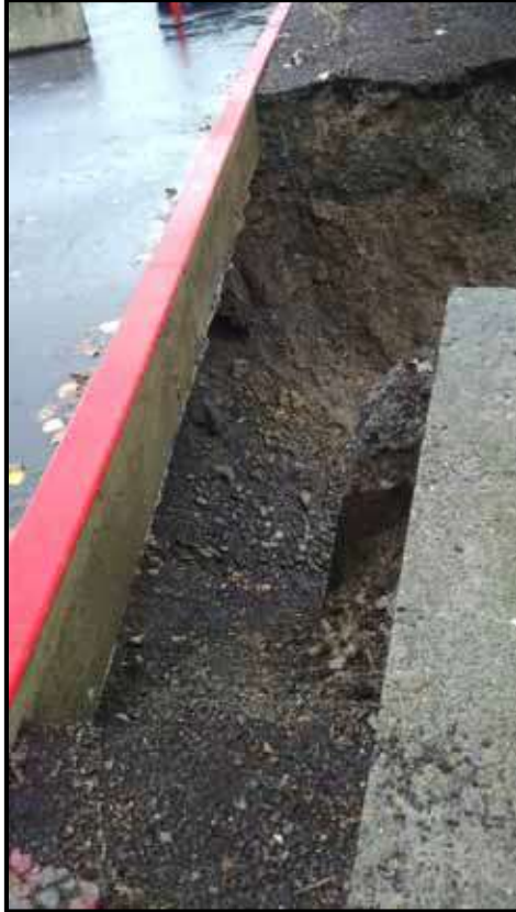
Unsupported pavement behind abutment wall from bridge
