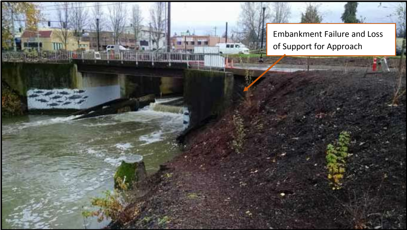
Facing northeast – overall bank erosion
