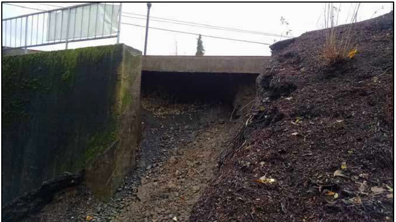
Unsupported pavement from below
