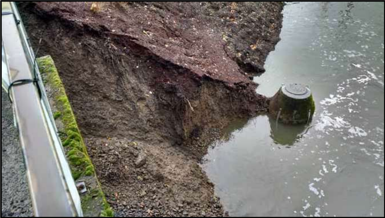
South abutment failure from bridge
