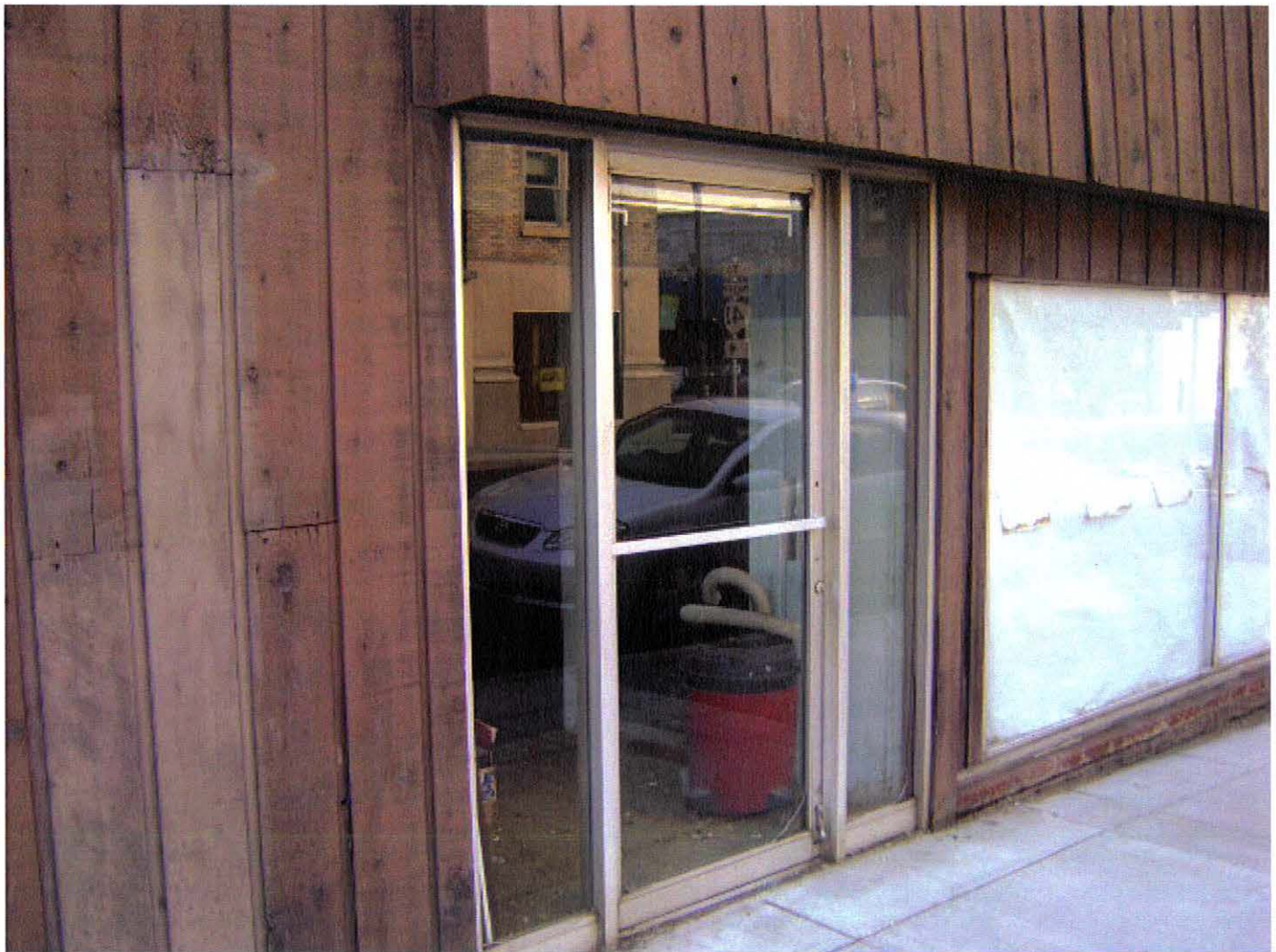
Recent site photos show existing conditions of building along 7th street facade, including weathered siding, damage to window base at corner, dated mansard detailing and aluminum entry door.
