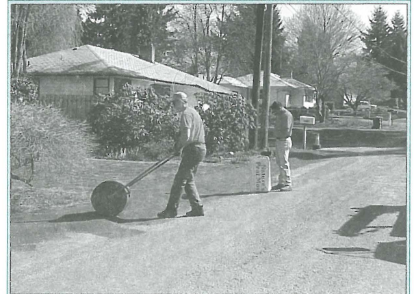
City workers construct some shoulder work to facilitate better drainage in Linwood.
