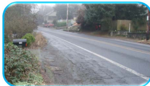
Pavement conditions in shoulder of Linn Avenue
