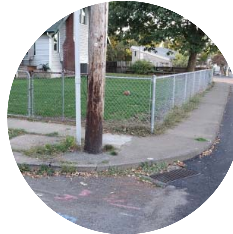
Intersections frequently lack curb ramps and other enhancements necessary for ADA compliance
