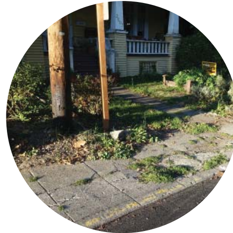
Sidewalks in this section are deteriorating in the vicinity of Spring Creek
