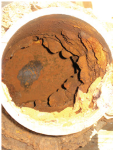
Some of Oregon City's water pipes are over 100 years old.
