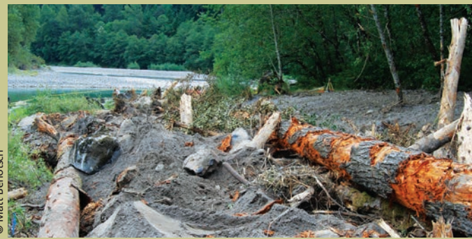
Construction of the log jam at the outlet of Happy Creek on the Sandy River in Oxbow Regional Park.
