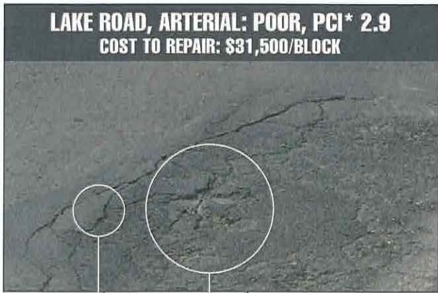
Cracks due to aging. Large holes due to aged asphalt, poor base material and sub-base failure. Base failure creates soft spot that is pushed down by traffic.
