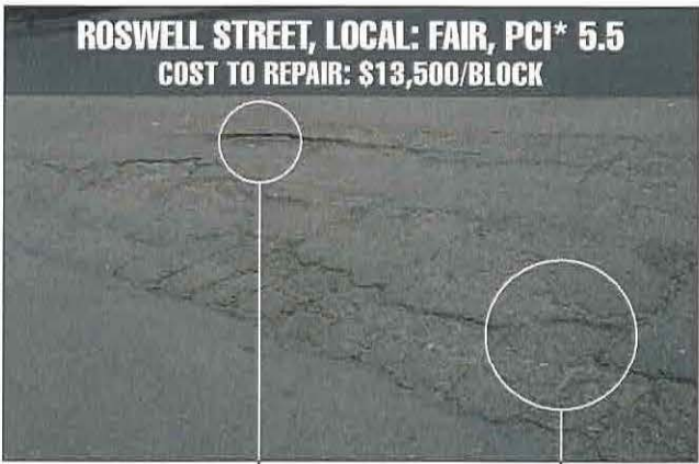
Water enters sub-base through cracks and, over time, the asphalt becomes brittle and breaks away. "Alligator" cracks caused by heavy vehicle traffic on aged asphalt.
