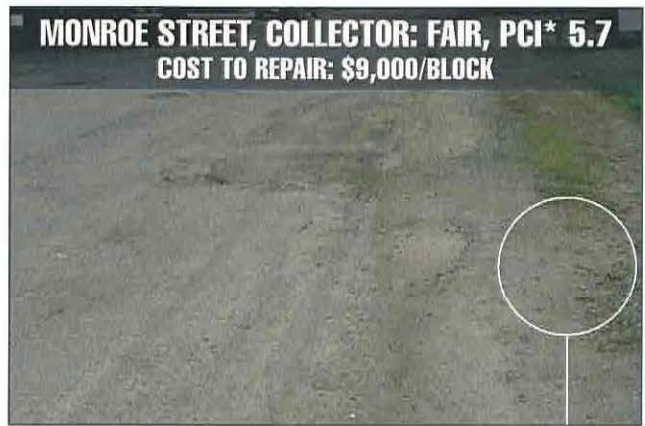
Poor shoulder drainage contributes to deterioration of aging asphalt. As asphalt is eroded, gravel is exposed and released.
