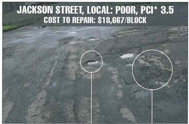
Poor drainage allows water to saturate base and sub-base. Roadway releases gravel from asphalt mix.
