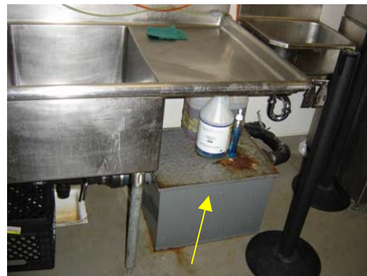
Example of a working retrofit grease trap
