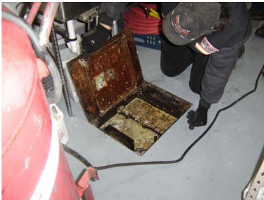
Example of a working in-ground grease trap
