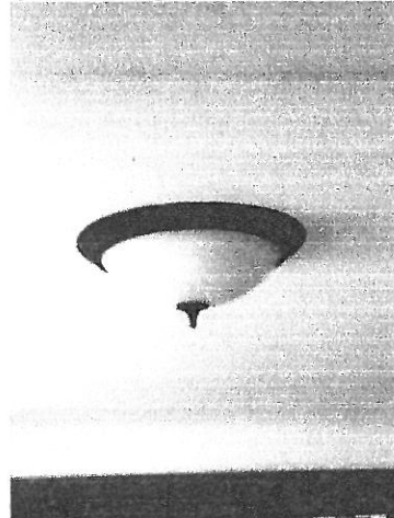
(Office Lighting) After:
