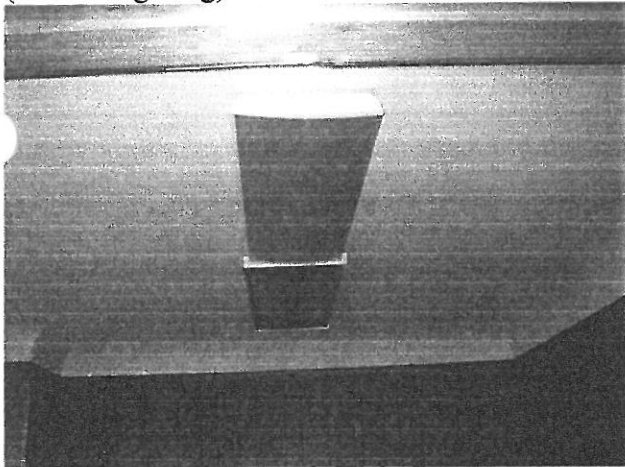
(Office Lighting) Before:
