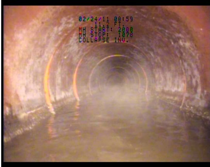
A snapshot from the video inspection of a undamaged section of the same pipe.
