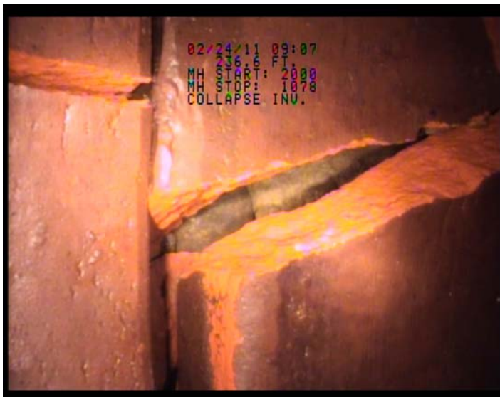
A closeup of a crack on the top of the pipe. Beyond this point TV inspection is not possible due to depth of flow.
