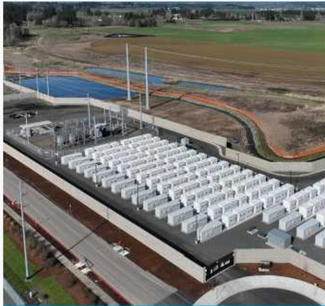
Bolstering reliability with local Battery Energy Storage System projects
